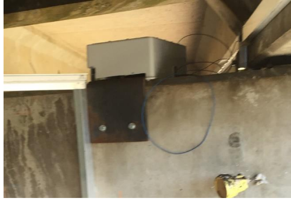
Figure 7: Junction Box Fitted Over Headstock Clamps
