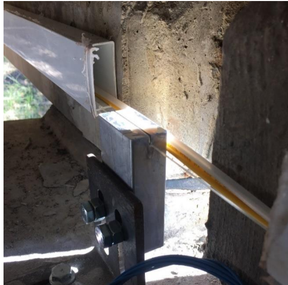
Figure 5: Longitudinal Sensor Cable Ducting
